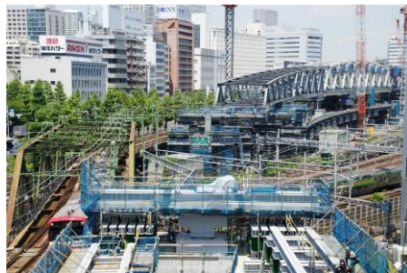
Replacement of the Yatsuyama Bridge between Shinagawa and Kita-Shinagawa on the Keikyū Main Line, spanning 10 JR lines
